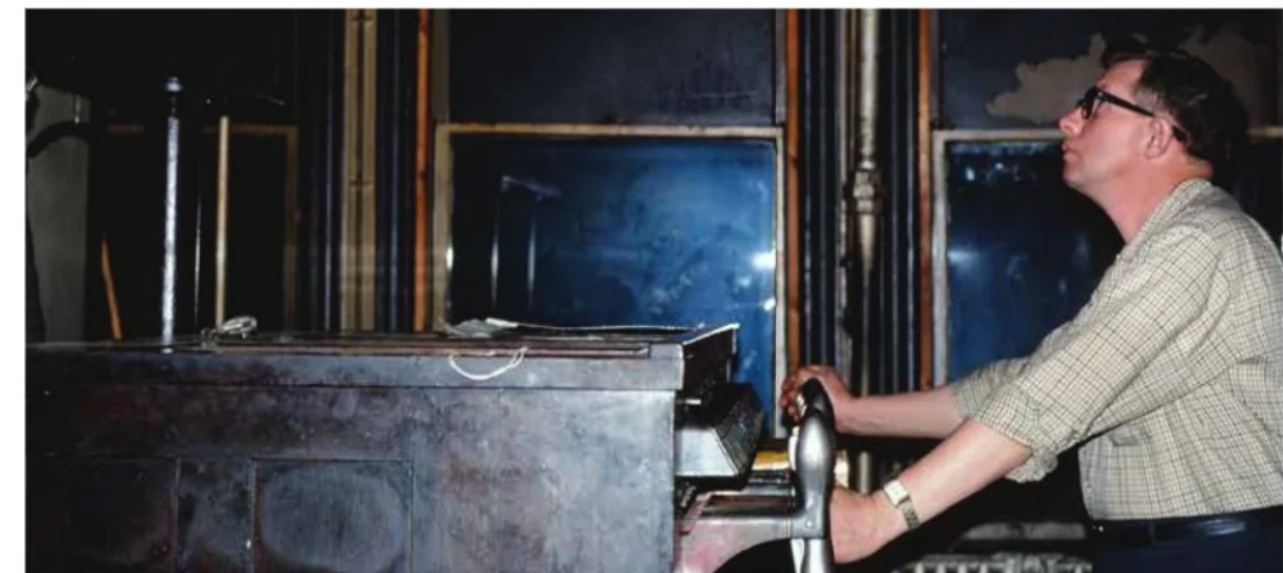
A towerman watches the progress of a train through the Athens Tower interlocking plant on a lighted occupancy board out of the camera's view. He'll pull the electrically actuated pistol-grip levers to give the consist the proper routing. Robert Archer
